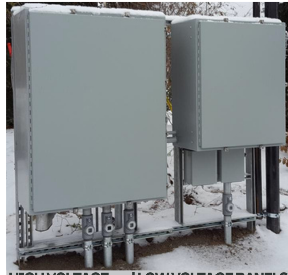
HIGH VOLTAGE and LOW VOLTAGE PANELS
